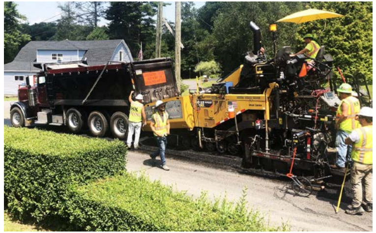
Shown moving slowly but progressively in the eastward lane towards Glen Lyon past the big curve in Lee are the crew and equipment of Pikes Creek Paving laying a coat of asphalt.
