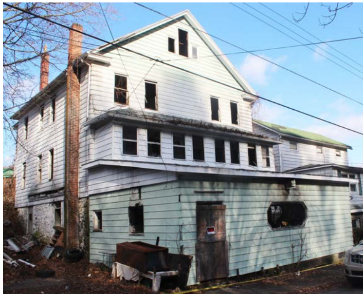
At near left is the property at 50-52 Newport Street which once housed Brexy's Bar. It had long been vacant when it caught fire last year and was significantly damaged. Please see Newport Township Community News , #70, Fall 2022, p. 15.
